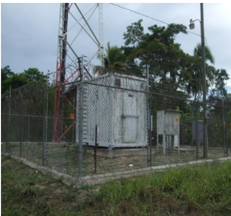
Figure A2 – 35. Telecommunications tower
